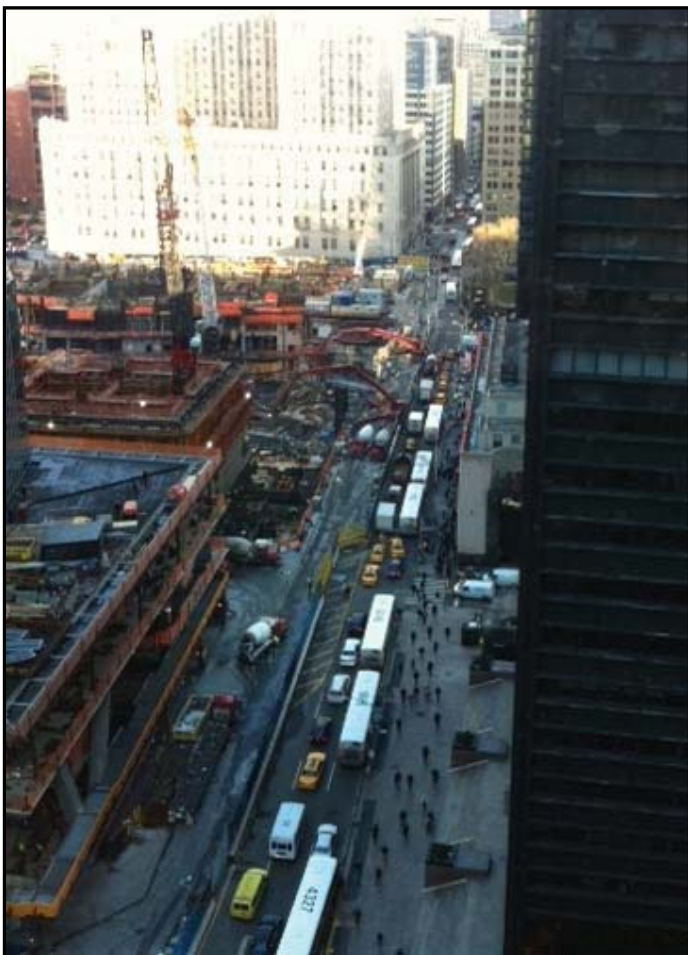
3. View north along Church Street with the World Trade Center Campus construction activities to the left.
