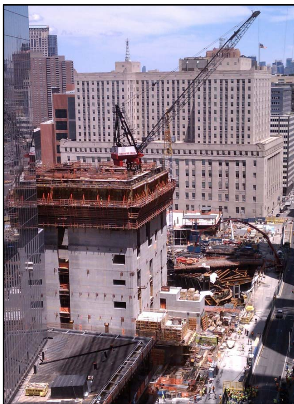
4. View of the WTC Campus from the south. The crane is located atop 3 World Trade Center.
