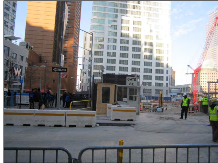
Photograph 6. The World Trade Center construction site west-adjacent to Greenwich Street between Cedar and Liberty Streets, view west.
