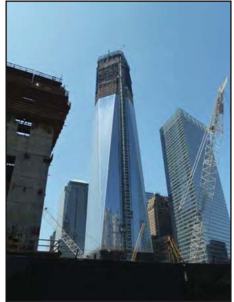
2. View of 1 WTC under construction facing west from Trinity Place/ Church Street.
