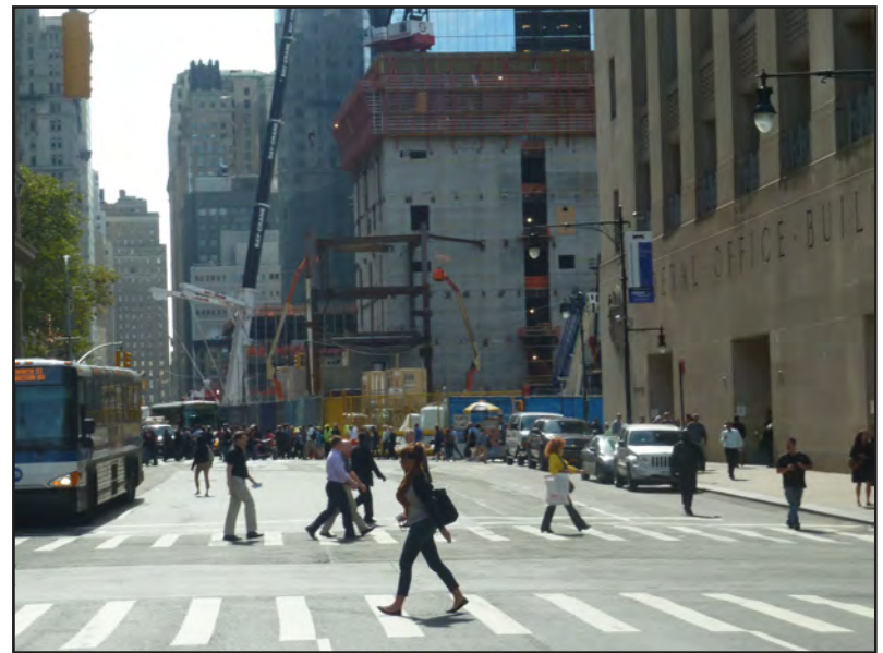
10. Existing view south along Church Street from a point north of Barclay Street.
