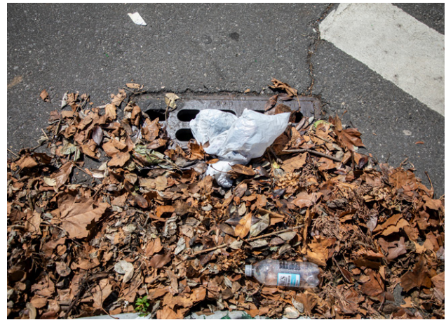
Debris on a storm drain.
